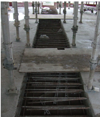
Pour Strips restrict site access, cause a trip hazard and delay progress on site
