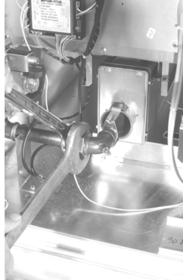
Figure 19 Disconnect gas manifold at the 90° elbow
