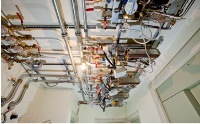
The picture shows Mini City substations mounted in a ceiling in the Zilverberg building.
