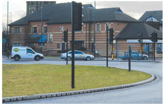
New ACO KerbDrain traffic islands which improve the flow of traffic at arterial junctions have been installed with minimal disruption.
