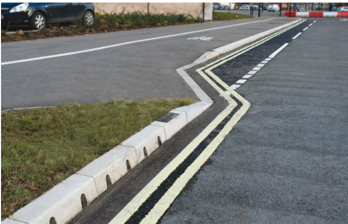
KerbDrain drop kerbs and flush centre stones have been used to integrate new cycle paths into the ring road highway network.
